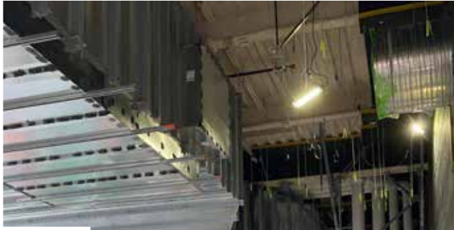
LEFT: One of the outside air ducts coming off of AHU-601. It is 142x72 with 1" liner.
